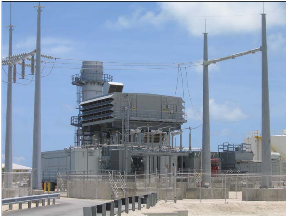
Combustion Turbine #4 at KEYS' Stock Island Generating Facility.
