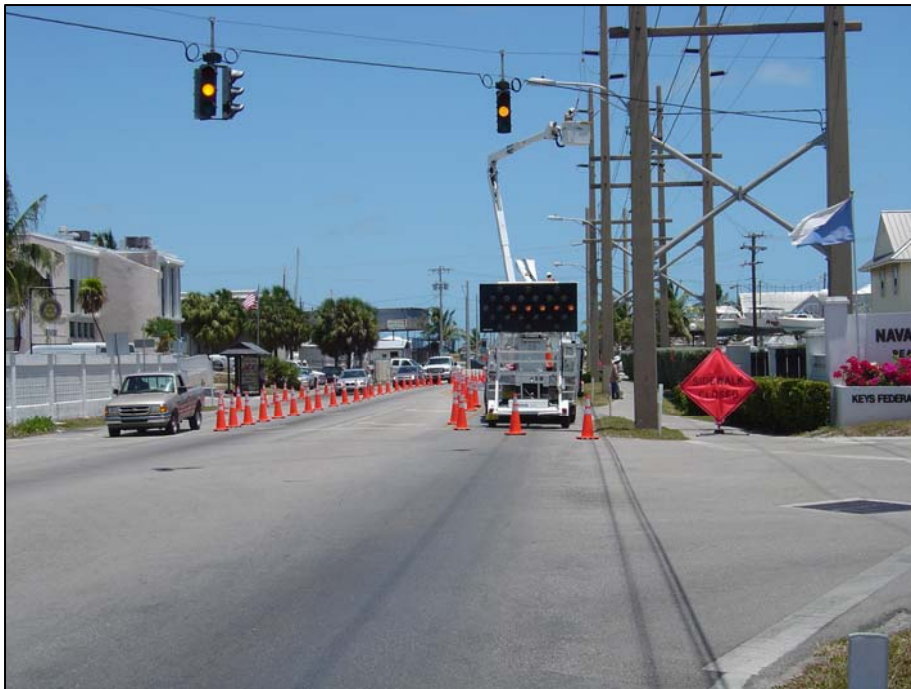
KEYS' Transmission & Distribution department employees work on system improvements on Palm Avenue in Key West utilizing proper maintenance of traffic procedures.
