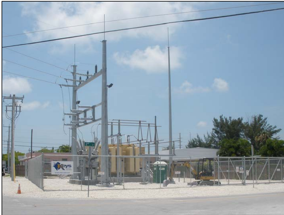
Second Street Substation in Stock Island.
